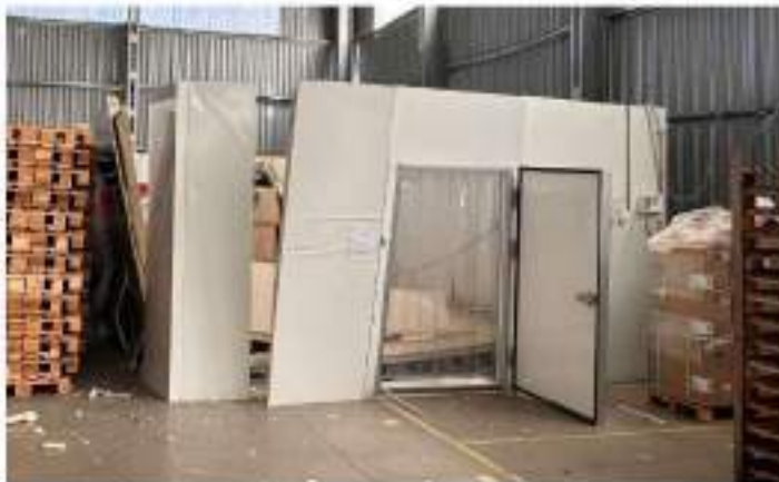
Damaged temperature-controlled room at Odesa warehouse.
