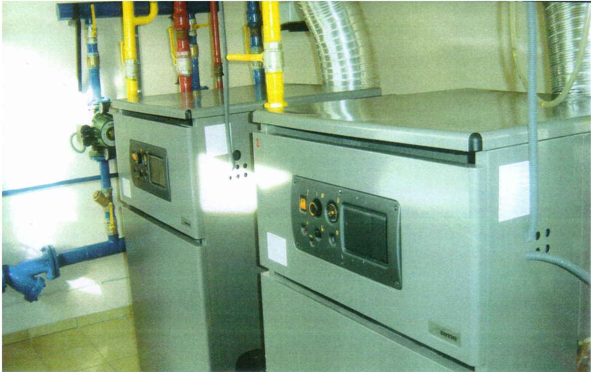
Series of activities at the Komrat province, Gagauzia region. Provision & installment of autonomus heating systems for Health Centers & Nursury Schools. Financing: HELLENIC AID Implementation: YPESDDA M O L D O V A
